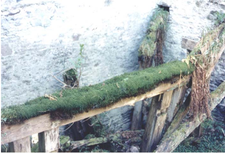
Decaying interior at Holemill 1988
